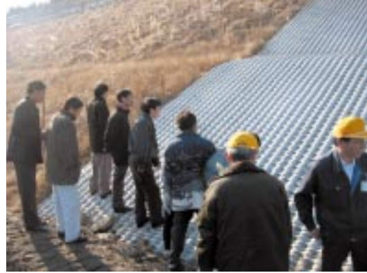
Slope covered with rubber sheeting to prevent leachate from seeping out of the landfill
