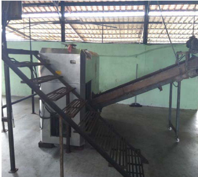
OWC Plant at Shakthan Nagar Thrissur
